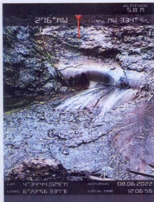
Fig D. SPILL POINT DURING EXCAVATION
